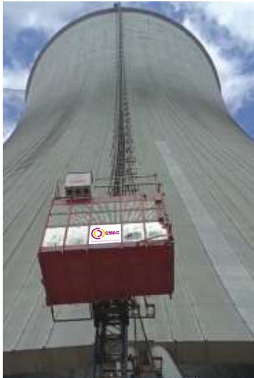
Curved Hoist RNPP, Bangladesh
