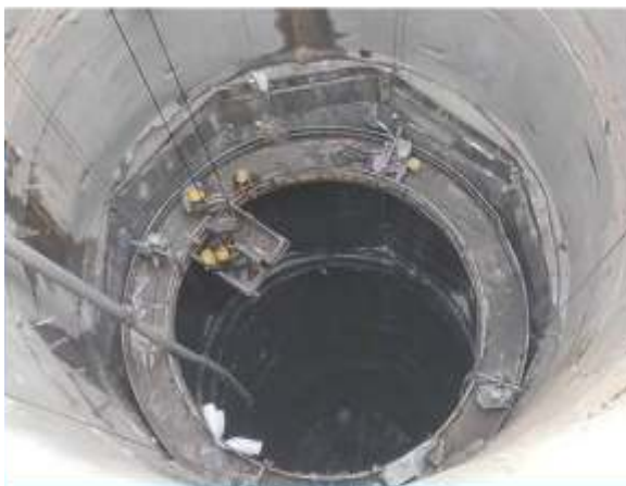
Circular Platform for Chimney/Vertical Duct Shaft at Kaleswaram
