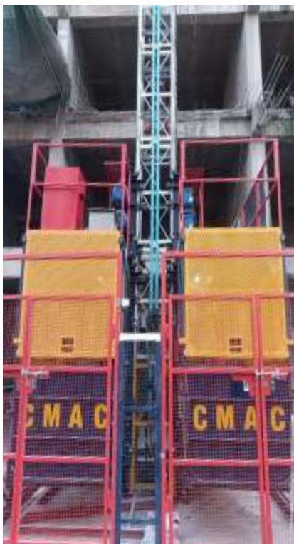
PM Hoist Double Cage ASBL | Runwal Group | Sweta Estates
