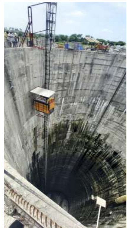
PMH at Pump House
